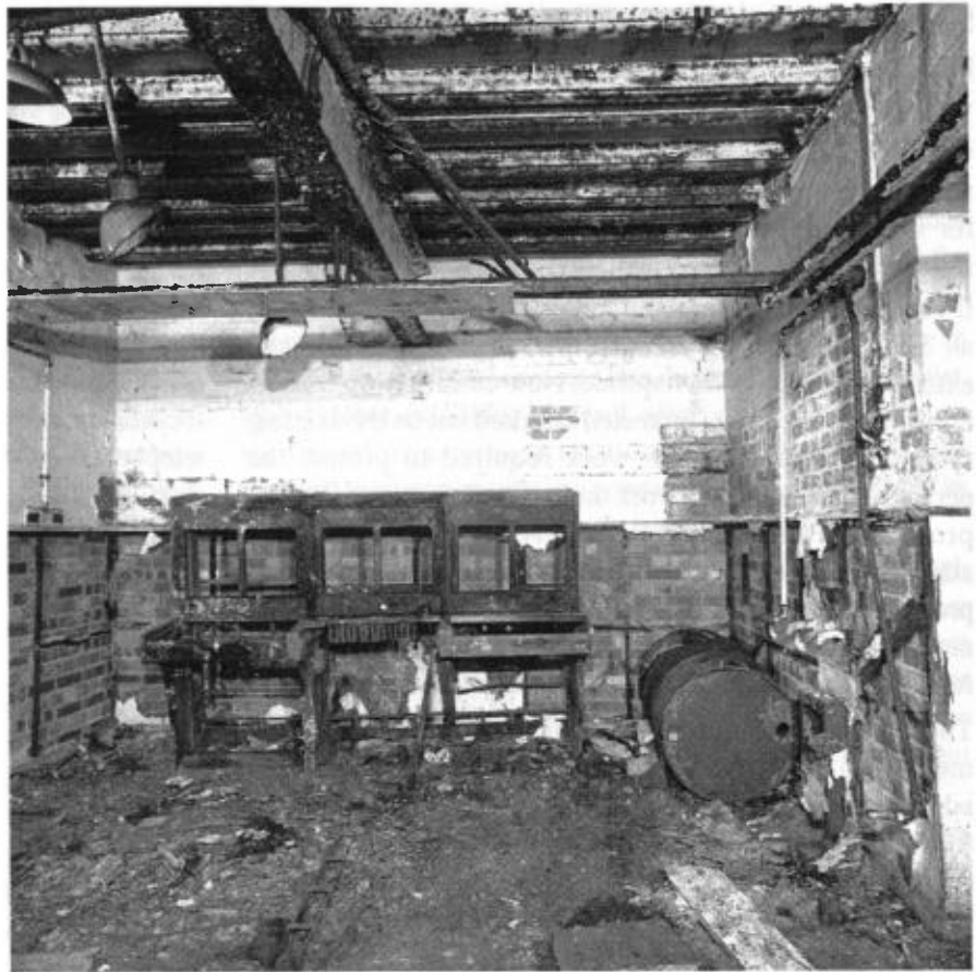
Deepdene; The three switchboards
